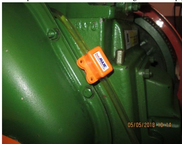
Figure 4.1: Fuel Line with 1 Magnetic fuel Energizer
