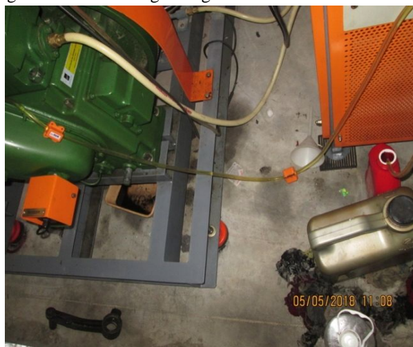
Figure 4.2: Fuel Line with 2 Magnetic fuel Energizer
