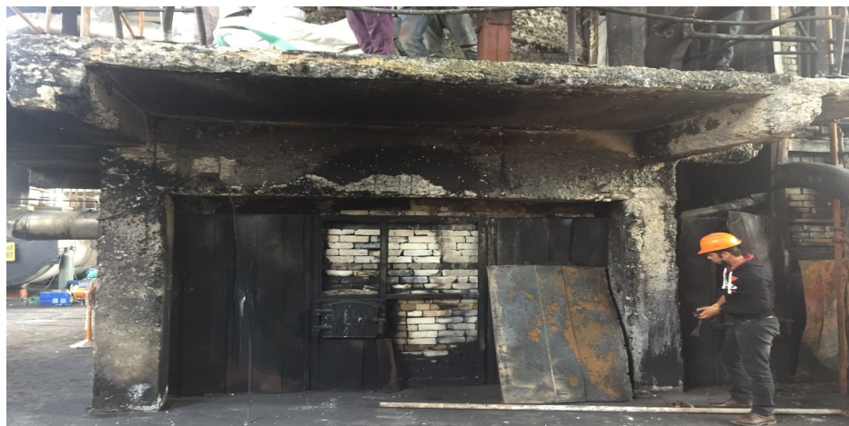
Figure 3 Fire hazardous fluid heating room at 1st Floor
