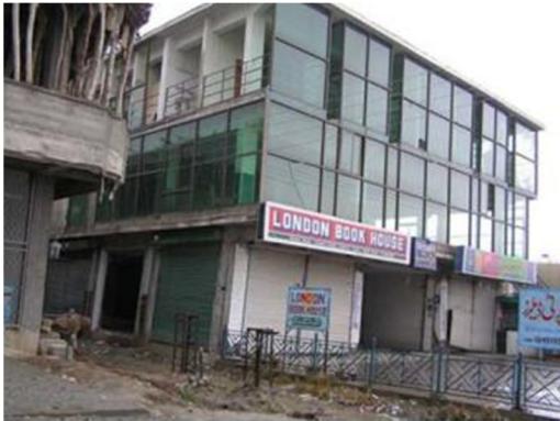
Fig. 2.1 Story failure of RC frames (Kashmir).
