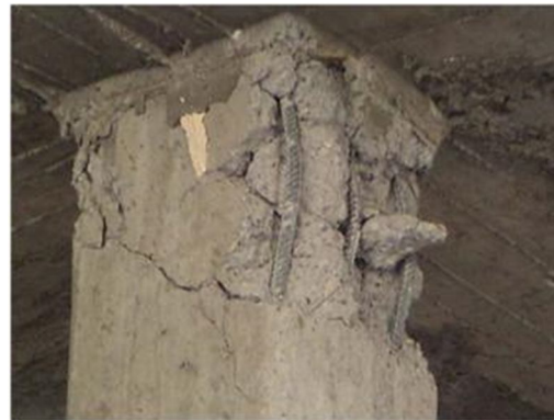
Fig. 2.5. The plastic hinge in a weak column (Iran).
