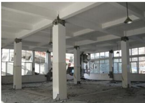
Fig. 2.3. Column damage (Wenchuan).
