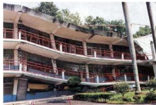
Fig. 2.6. Collapse of school (Taiwan).
