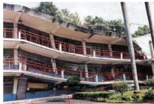
Fig. 2.6. Collapse of school (Taiwan).
