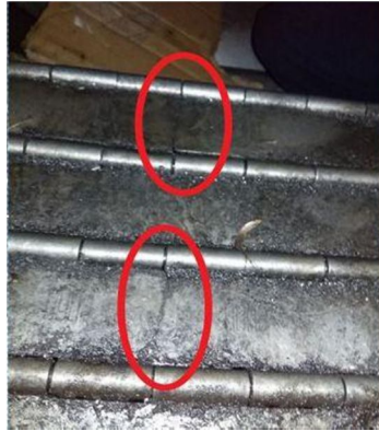
Fig. 13 Sheared Hinge Plate & Bent Hinge Plate
