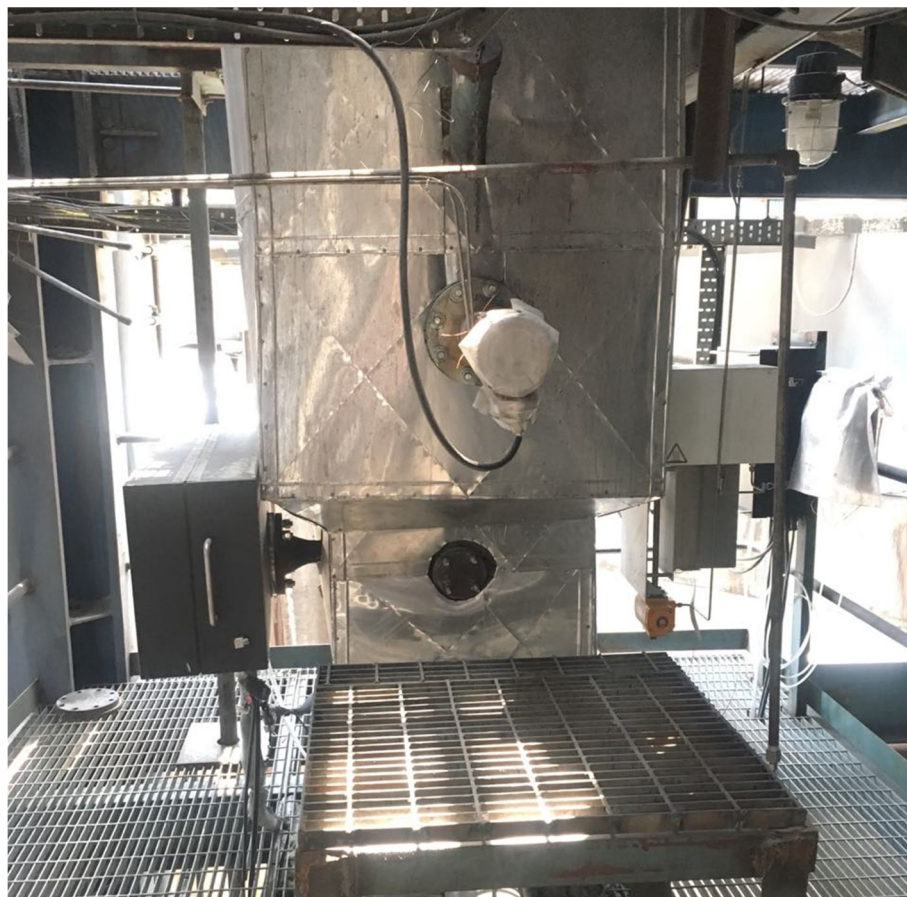
Fig: 5 Catalyst at thermal power plant
