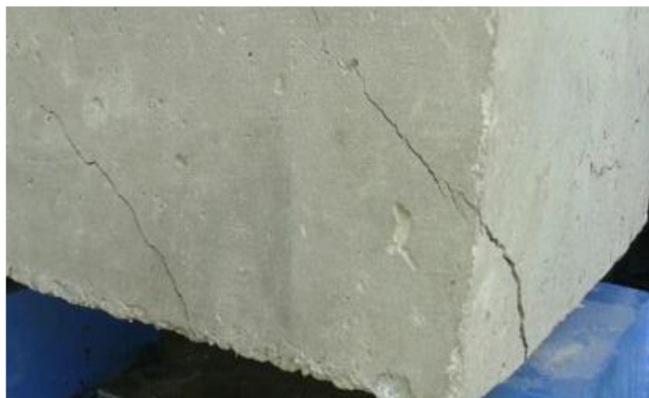
Fig .2 Cracks in bubble slab
