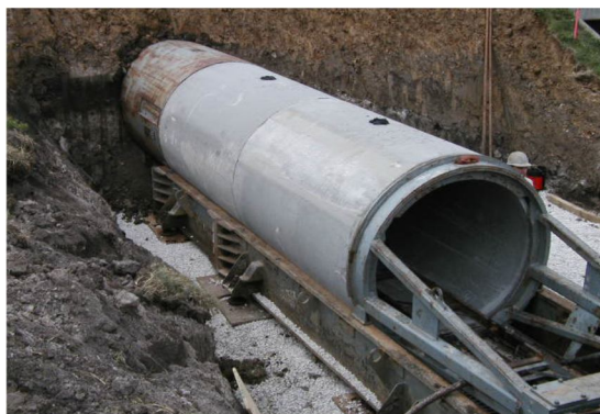
Figure 2.3. Concrete pipe being jacked into place behind cutterhead assembly fixed with . For spoil bucket removal to out of pipe for track leading
