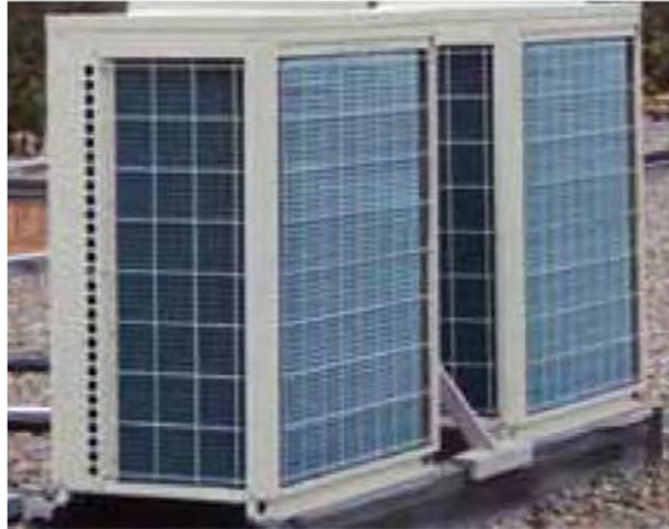
Figure 1.2: Two outdoor condensing units installed on a rooftop
