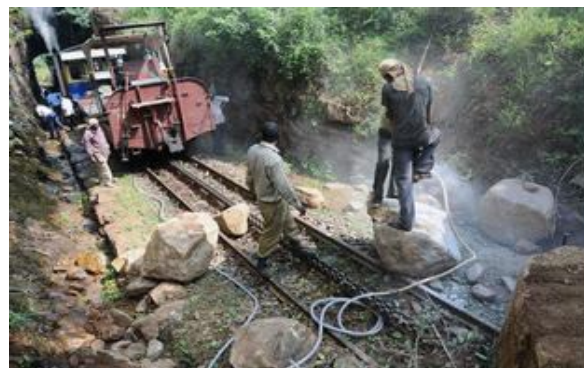
Fig. 2 Blockage of the rail road
