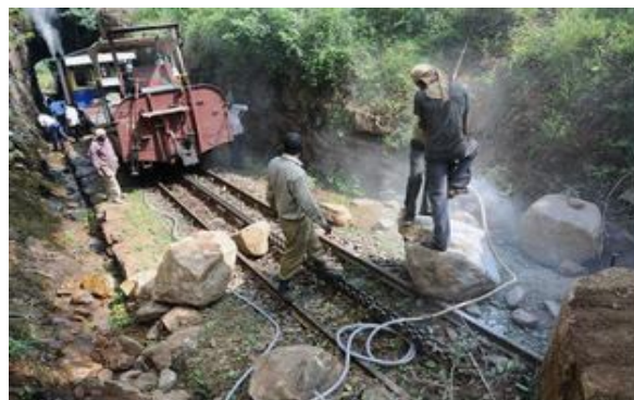
Fig. 2 Blockage of the rail road
