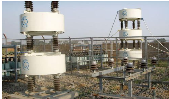
Fig: Air Core Dry Type Reactor
