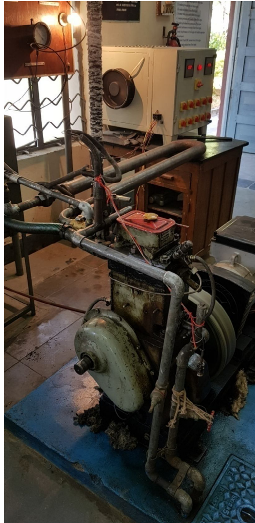
Fig 3: Diesel engine with heat exchanger
