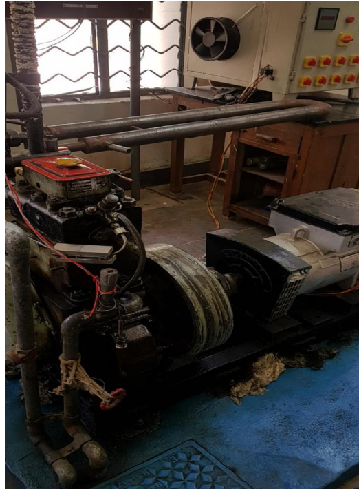
Fig 5: Diesel engine with magnet and EGR
