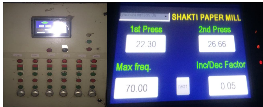
Figure 3.2 HMI with PLC
