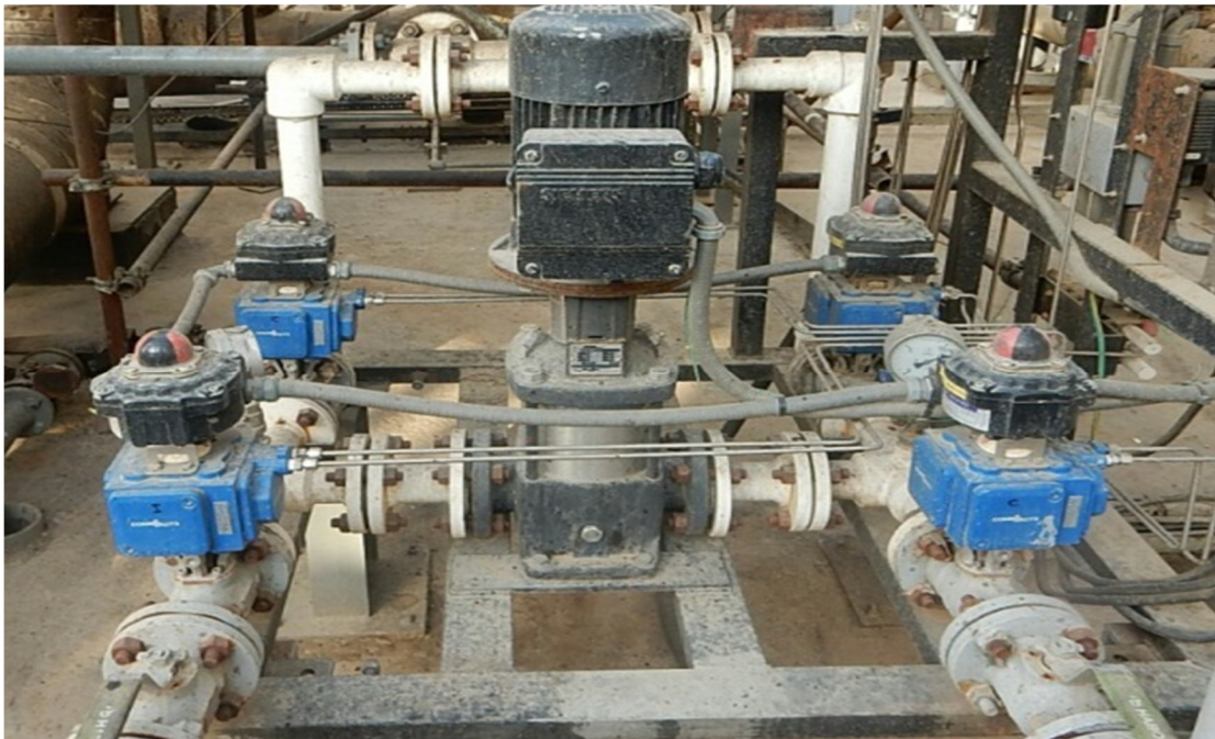
Figure 1: ATCS unit used for experimentation
