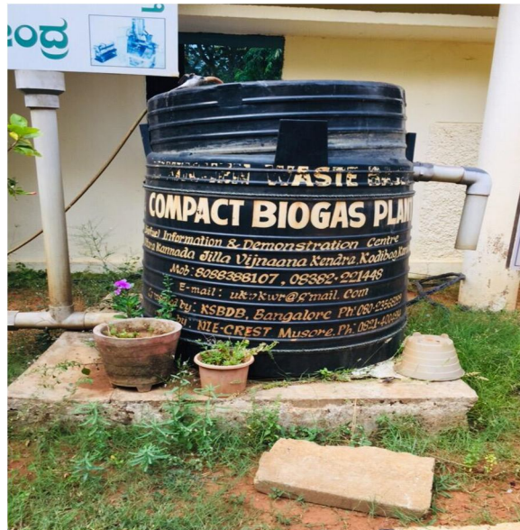
Fig-7 Biogas plant in Science centre karwar.
