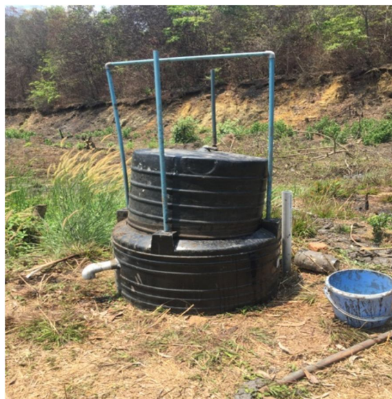
Fig-9 Installing biogas plant with a capacity of 750lts in Girijabai Sail Institute of Technology is in progress.
