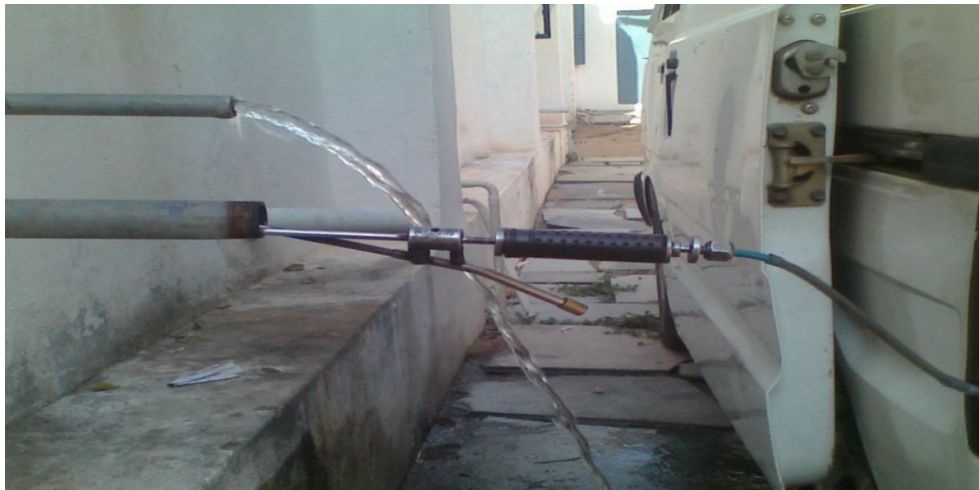
Fig 10. Closer View of Emission Test Unit Connected To Engine Exhaust Valve
