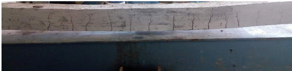
FIG NO. 1: Crack pattern in rectangular beam
