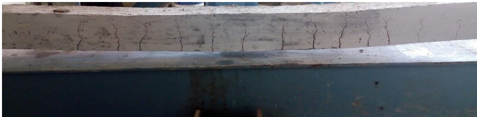
FIG NO. 1: Crack pattern in rectangular beam
