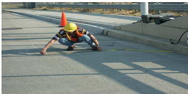
Figure-1: Manual Inspection of Crack on Roads
