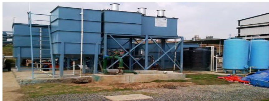
Fig 6 Waste Water Treatment Plant
