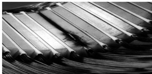
Fig.3. Motor winding damage due to ground fault
