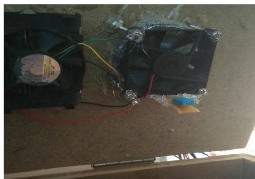
Fig 7 : Cooling and Heating unit
