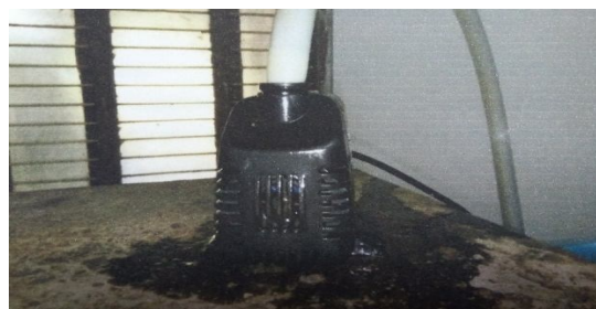
Fig. 4. pump for de-humidifier
