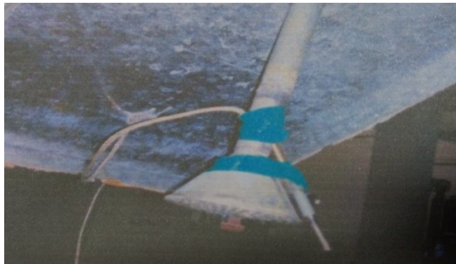
Fig. 7. humidifier section with thermocouple
