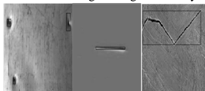
(Fig.D With the help of Boundary Box Algorithm Defects are covered)
