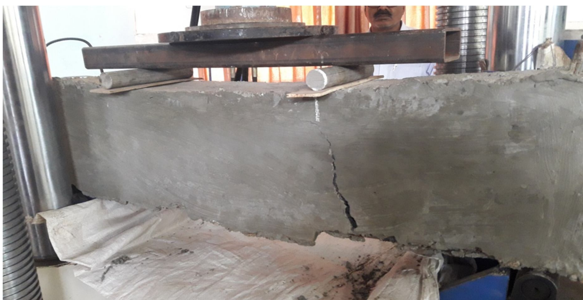
Figure-13 Crack width of control beam.
