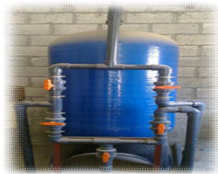
Fig: 1b. Saline Water Tank
