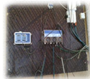
Fig: 2b. Automatic Fertilizer Mixing Control Panel
