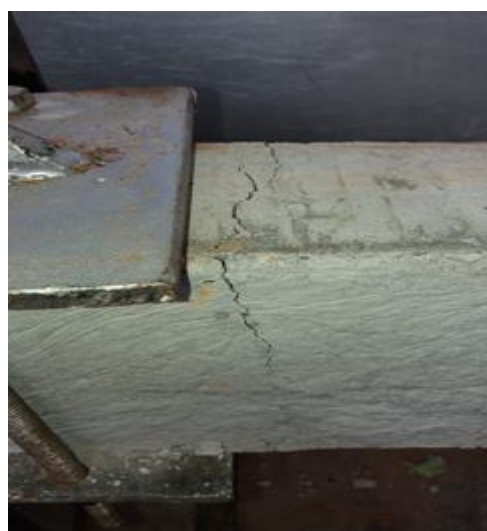
Figure: (4) cracking in beam.
