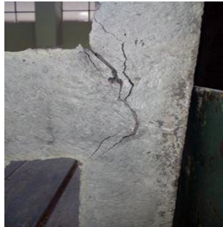
Figure: (6) Joint shear failure.
