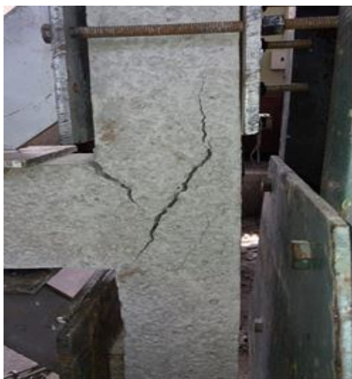
Figure: (3) cracking in joint.
