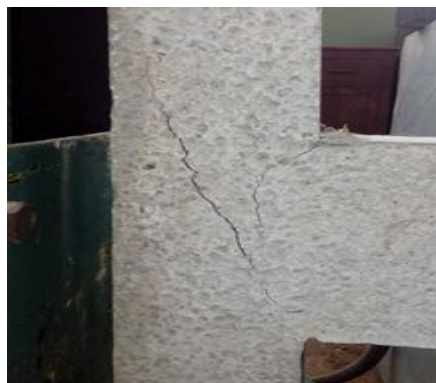
Figure; (2) Joint shear failure.
