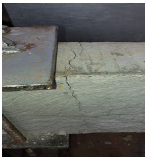
Figure: (4) cracking in beam.
