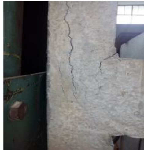
Figure 7: Joint shear failure.
