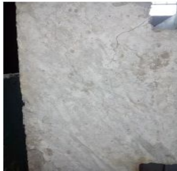
Figure 2: Interface and joint shear cracking.
