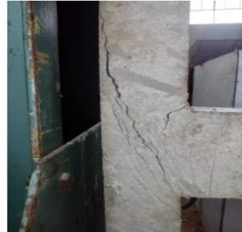
Figure 3: Joint shear failure.
