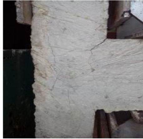
Figure 5: Joint shear cracking.
