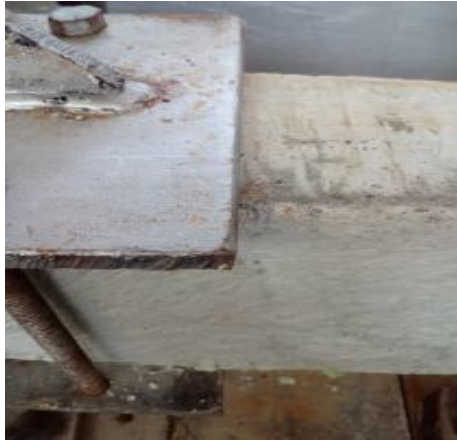
Figure 4: Beam flexure cracking.
