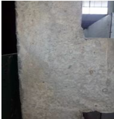
Figure 6: Initiation of cracking.
