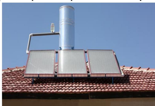
Fig-1: Solar water heater system
