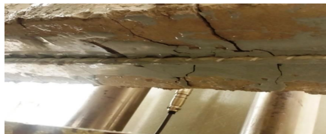
Figure 10 Debonding of GFRP rod
