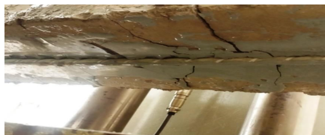
Figure 10 Debonding of GFRP rod
