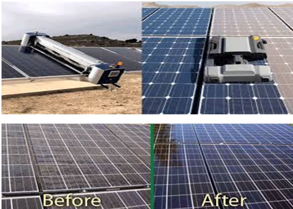
Fig-I Clean Solar panel and solar panel with dust
