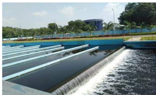
Fig.13. View of chlorine contact tank
