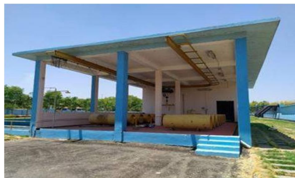
Fig.12. View of Chlorination unit
