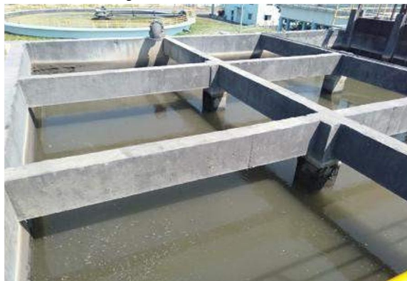
Fig.2.Inlet chamber of STP
