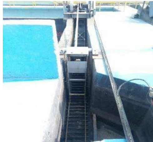
Fig.5. View of mechanism of grit separator (Rack classifier)
