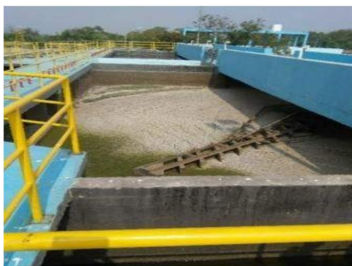
Fig.4. Showing the inner view of grit removal
