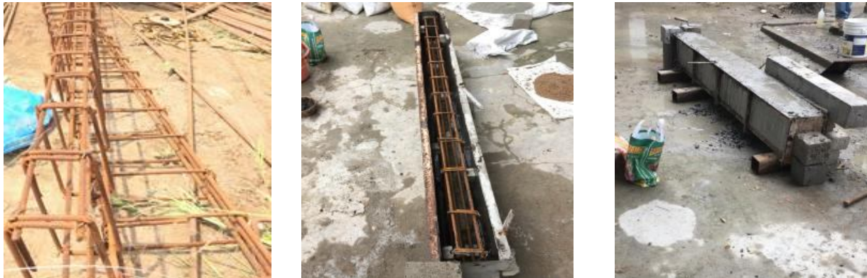
Fig 8. (a) Tying of reinforcement cage; (b) reinforcement in casting box; (c) casting of beam
