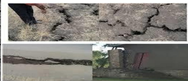
Fig 3 : Cracks on pavement and building constructed on Black Cotton Soil
