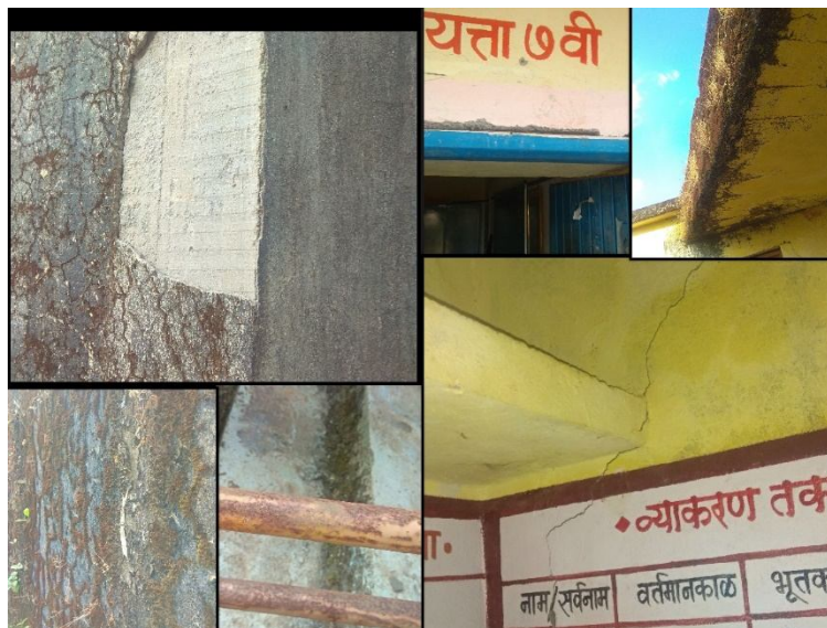
Fig.5 Defects in Warewadi
