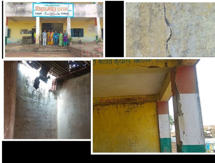
Fig.2 Defects in Charan
