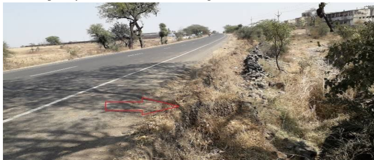
Figure 3:- steep embankments at near dondwada village.
