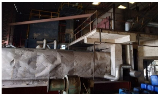
Fig 2: Briquette Boiler in Plant
