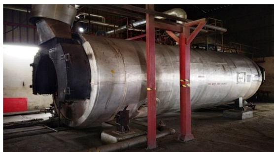
Fig 3: Furnace Oil Boiler
