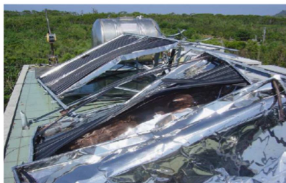
Figure 1: Solar panels damaged due to strong winds in Taiwan
