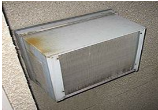
Fig.1; Air conditioning Equipment
