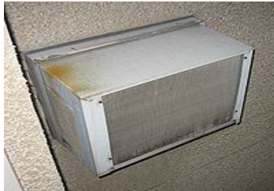
Fig.1; Air conditioning Equipment
