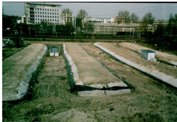
Fig. 3. View of the remediation facilities with the piles, service containers and bioreactors
