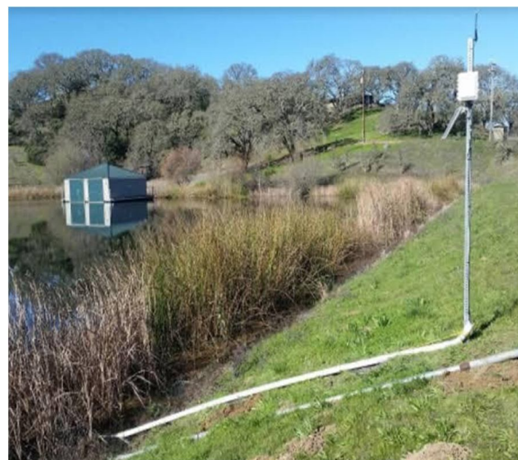
Actual Image of Water level Sensor.
