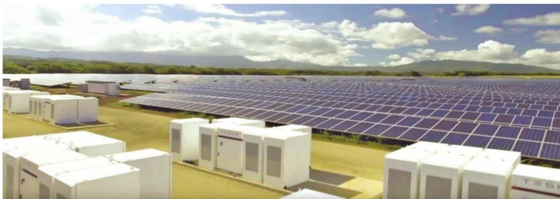
Fig. 2. Solar Photo Voltaic System
