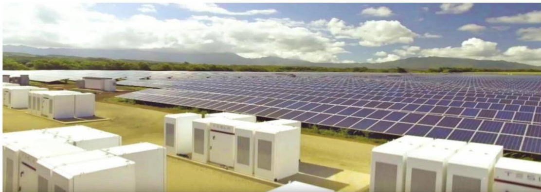
Fig. 2. Solar Photo Voltaic System
