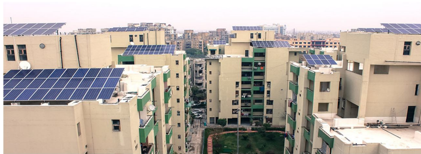
Fig 2 roof top solar system
