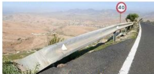
Damaged Steel barrier
