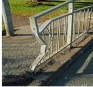
Damaged steel barrier
