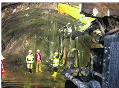
Fig 4: Water ingress at the last point of the excavation
