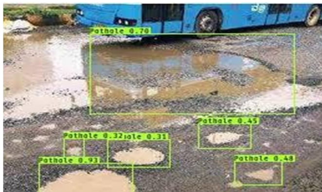
FIG: Pothole Detection 1
