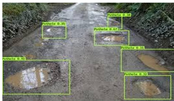
FIG: Pothole Detection 3
