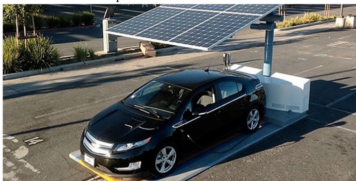
Figure 1:Solar Electric Charging Station
