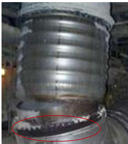
Figure-2: Failed Expansion Bellow
