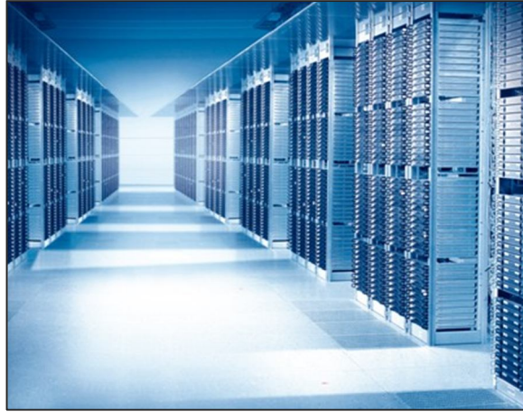
Fig 6: Cloud Storage Server
