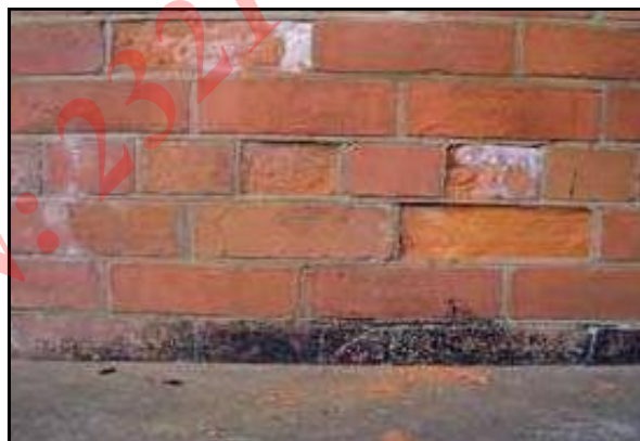
Photo No. 1. Affected Wall by Salinity
