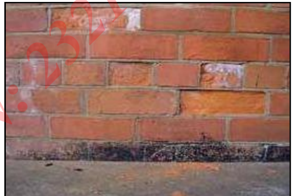
Photo No. 1. Affected Wall by Salinity
