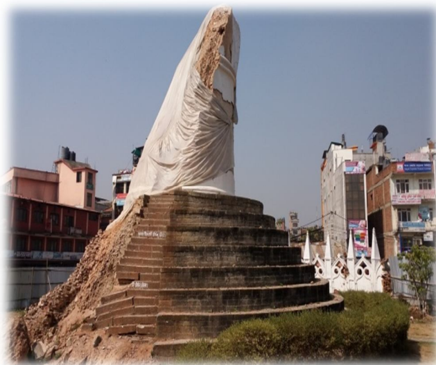
Figure 1: damaged dharahara tower, kathmandu
