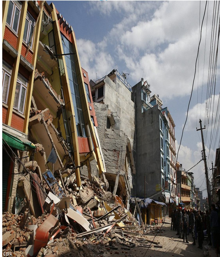
Figure 2: column, joints fail
