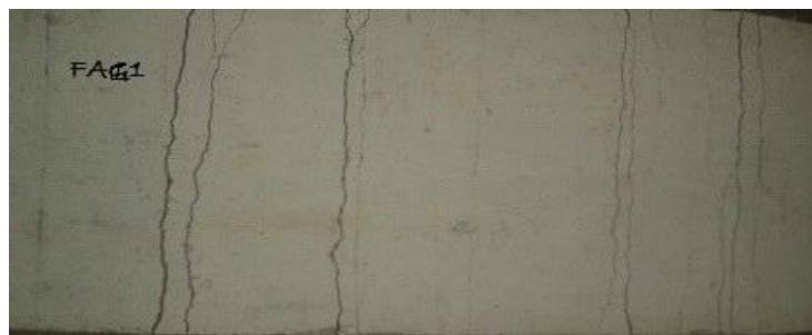
Figure 5.2 evenly distributed crack pattern in FCCG
